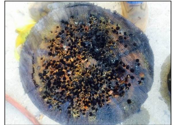
Pier 3 pile cross-section showing marine borer damage
